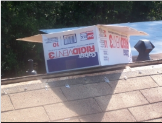
Gaf ridge shingle over vent
