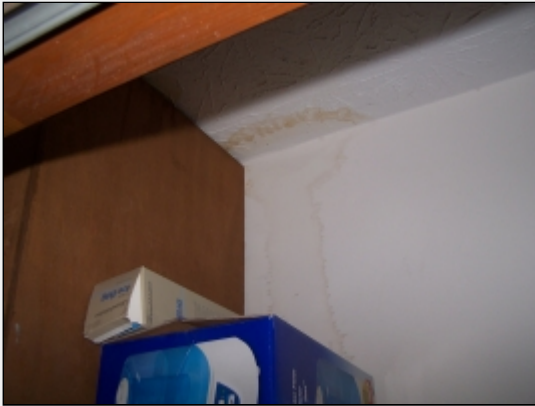
Water stain Closet
